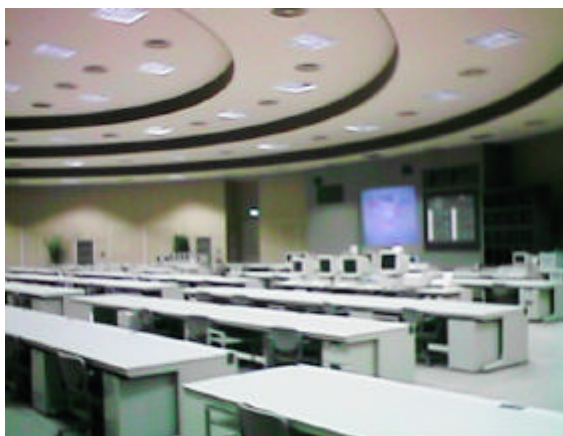
Fig.4 Central control system COCOS installed in the main control hall
