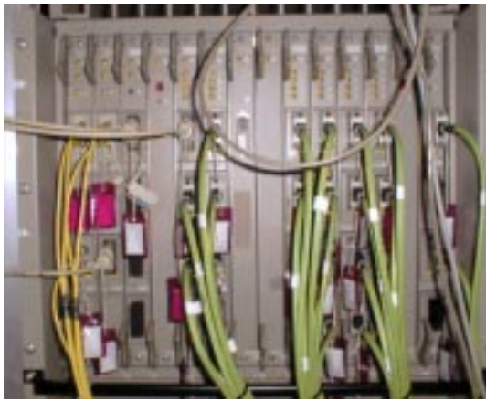
Figure 2. The front panel of the FDDI switch in the KEKB central control building. Each optical fibre cables are connected to the FDDI-Ethernet bridges in the local control rooms.
