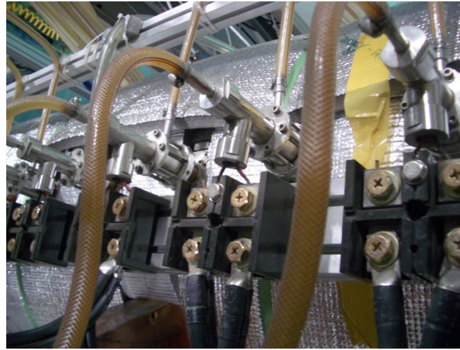
Air shower and general terminal block
