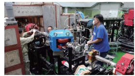
The inside of the vacuum chambers was wet with water and all chambers had to be disassembled.
